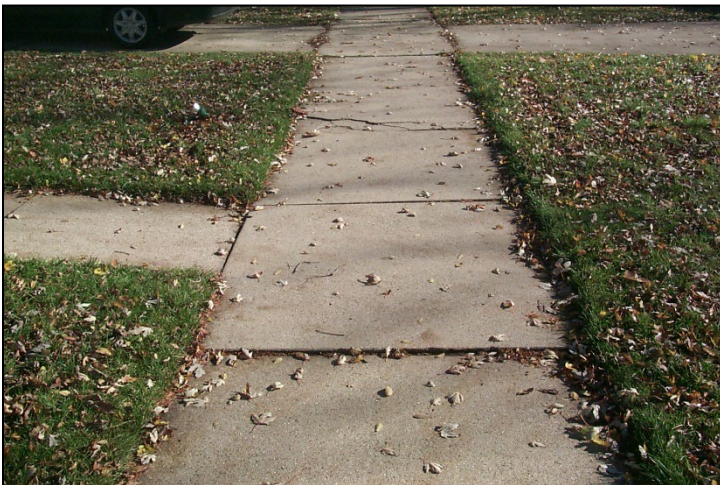
Figure 1 – Sidewalk Height Discrepancy
