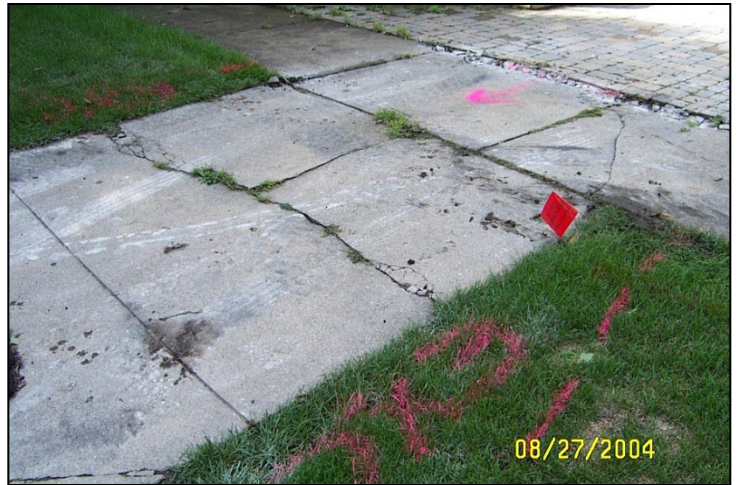
Figure 6 – Cracked Sidewalk and Apron
