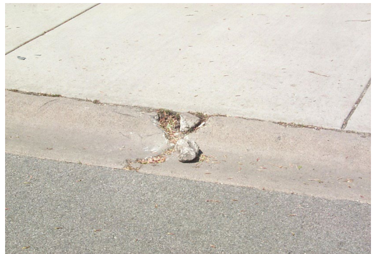
Figure 10 – Broken Curb, Concrete Apron
