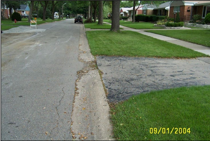
Figure 9 - Deteriorated Curb, Asphalt Apron
