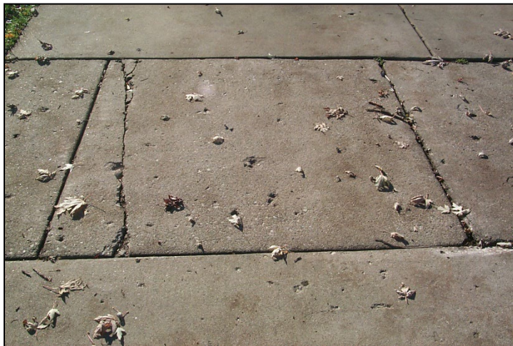
Figure 2 – Crack in Sidewalk
