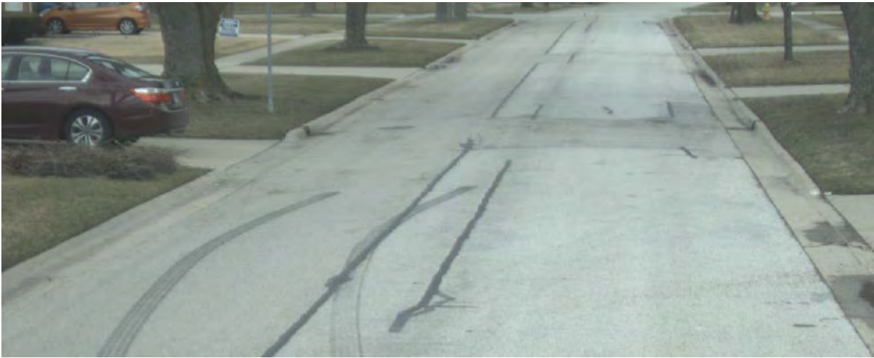
Figure 3-10: Leahy Circle Section 10, PCI 76 (Satisfactory)
