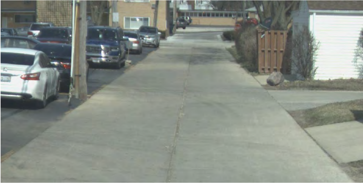
Figure 3-9: Broadway/Seventh Section A8, PCI 85 (Satisfactory)
