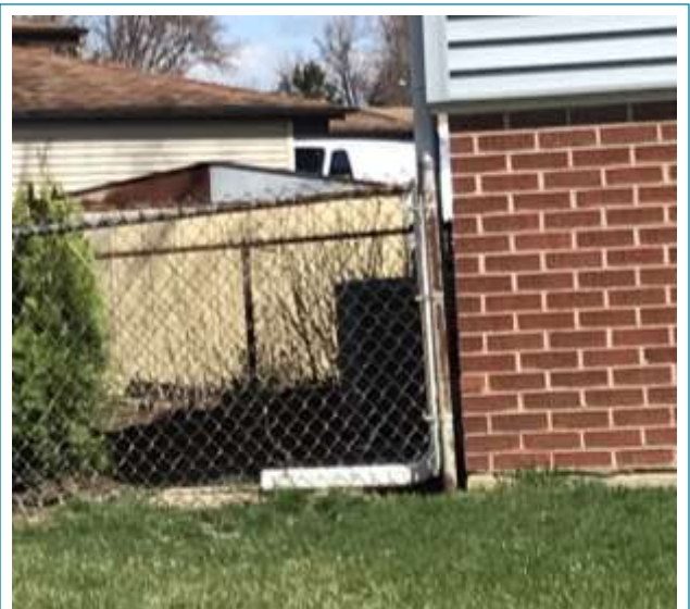
Figure 33. Typical Structure in Repetitive Loss Area 14. The owner of this property in Repetitive Loss Area 14 has a small extension on their downspouts and a splash pad. If seepage is a problem, a longer downspout extension would drain runoff away from the structure more efficiently.
