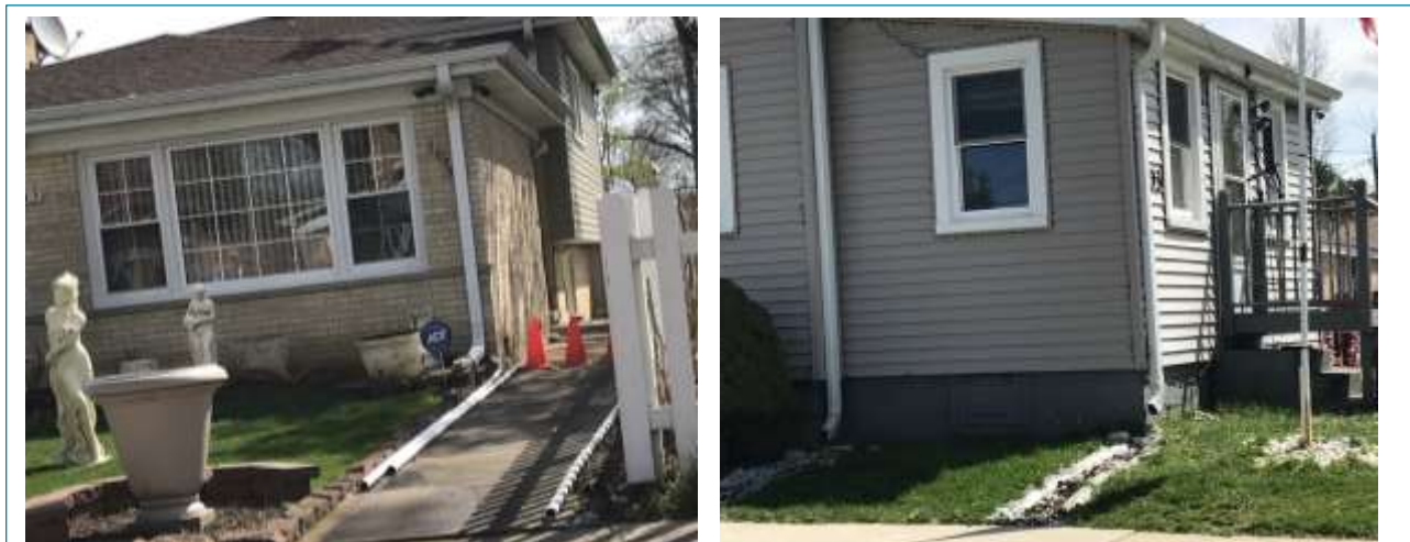
Figure 23. Typical building within Repetitive Loss Area 9. In the image on the left, the sump pump discharge pipes have been extended to allow positive drainage away from the structure. Another alternative, shown in the image on the right, is a stone swale sloped away from the structure.
