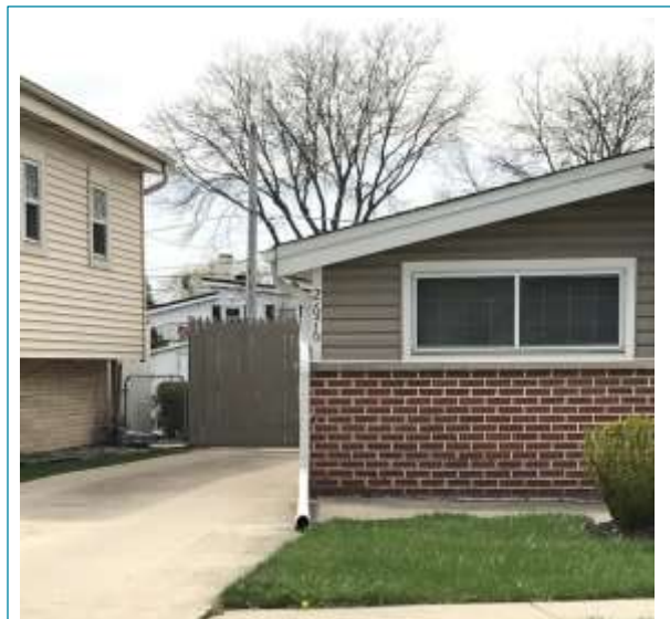
Figure 27. Typical Structure in Repetitive Loss Area 11. Many of the downspouts in this area have been extended; as shown in the above image.
