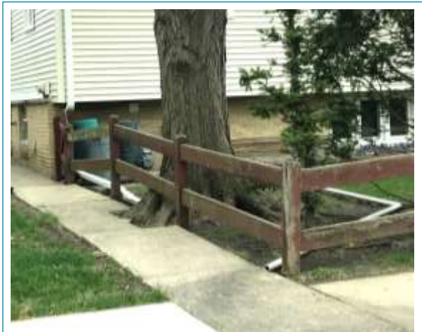
Figure 29. Typical Structure in Repetitive Loss Area 12. Many of the downspouts and sump pump discharges in this area have been extended; as shown in the above image.
