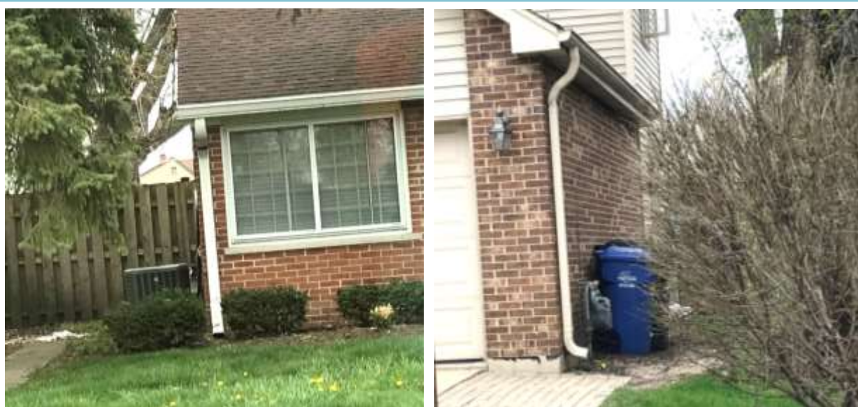
Figure 25. Typical downspouts in Repetitive Loss Area 10. As shown above, many of the downspouts within Repetitive Loss Area 10 were not extended. The majority of structures in this area do not have basements; therefore, seepage and continually running sump pumps may not be an issue.
