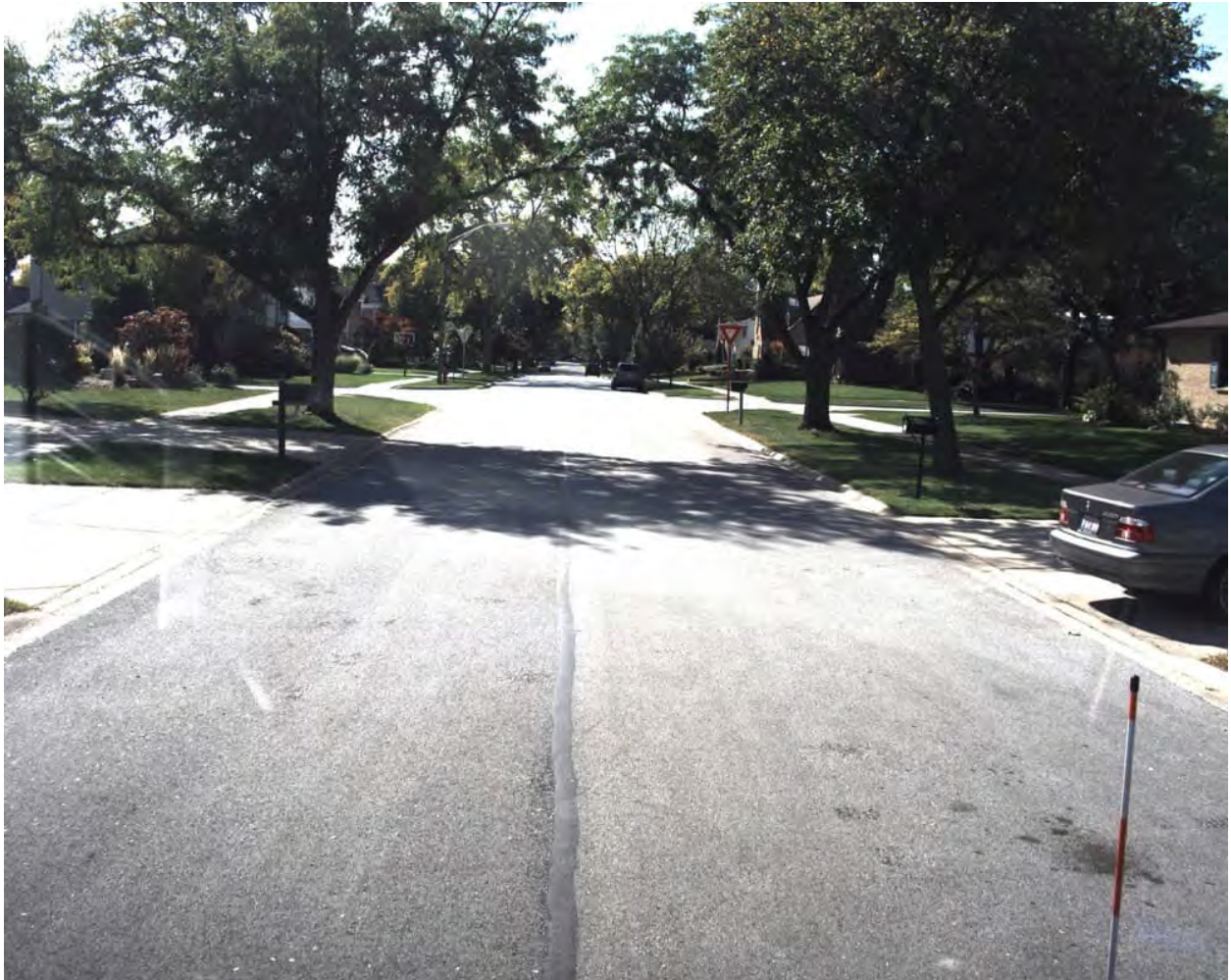
Figure 3-9: Ardmore Rd Section 00, PCI 84 (Satisfactory)
