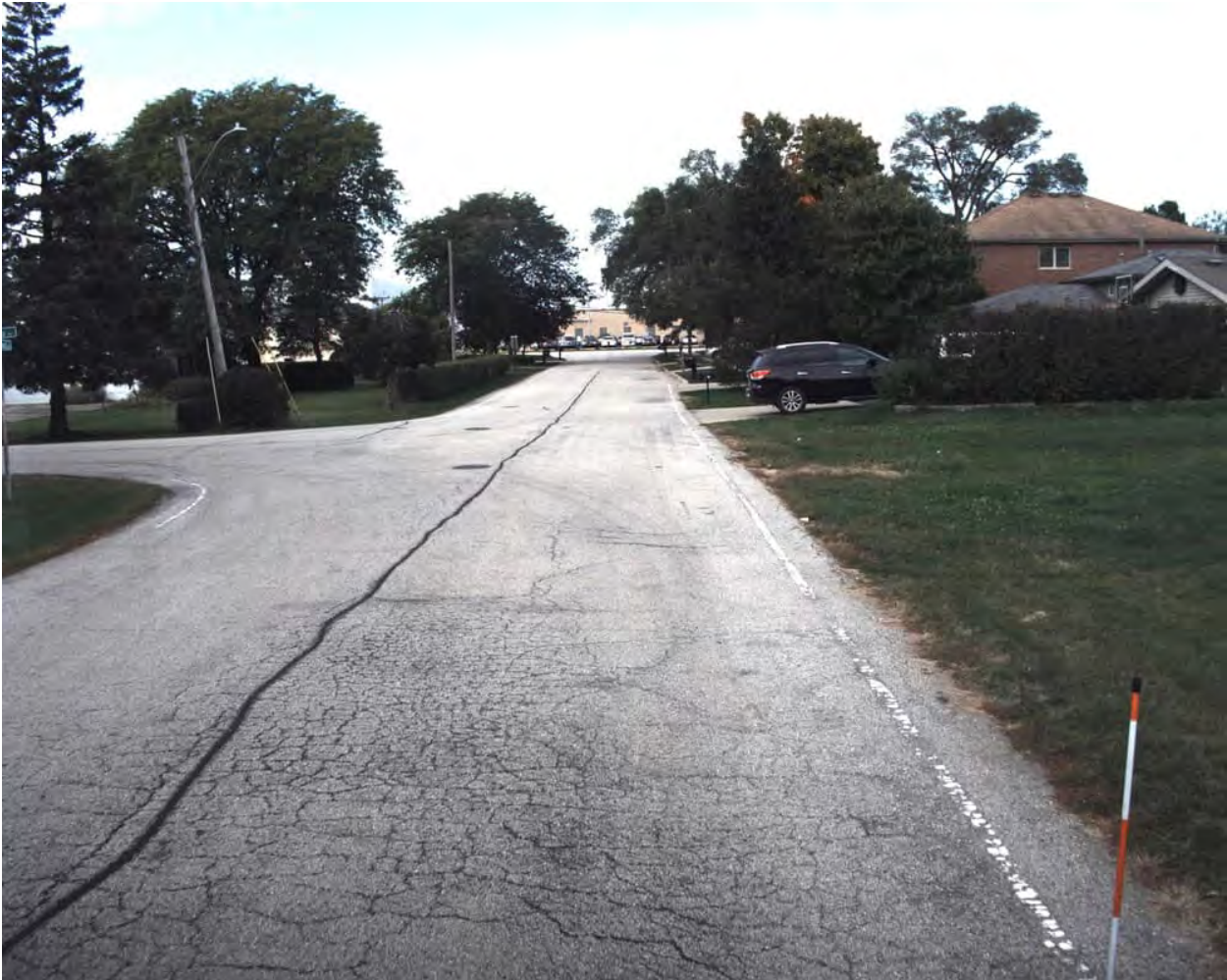
Figure 3-17: Birchwood Ave Section 00, PCI 30 (Very Poor)
