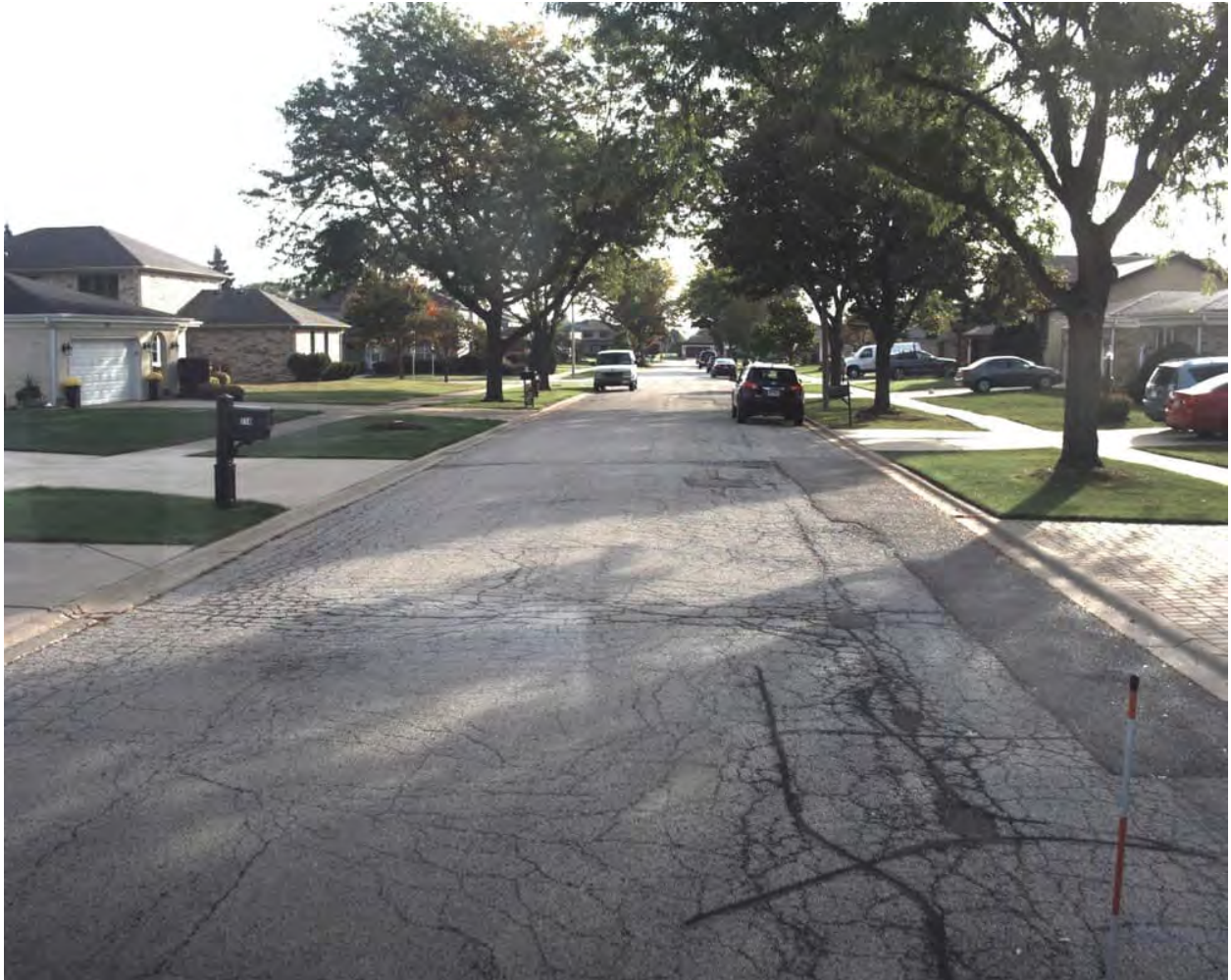
Figure 3-18: Yorkshire Ln Section 00, PCI 24 (Serious)
