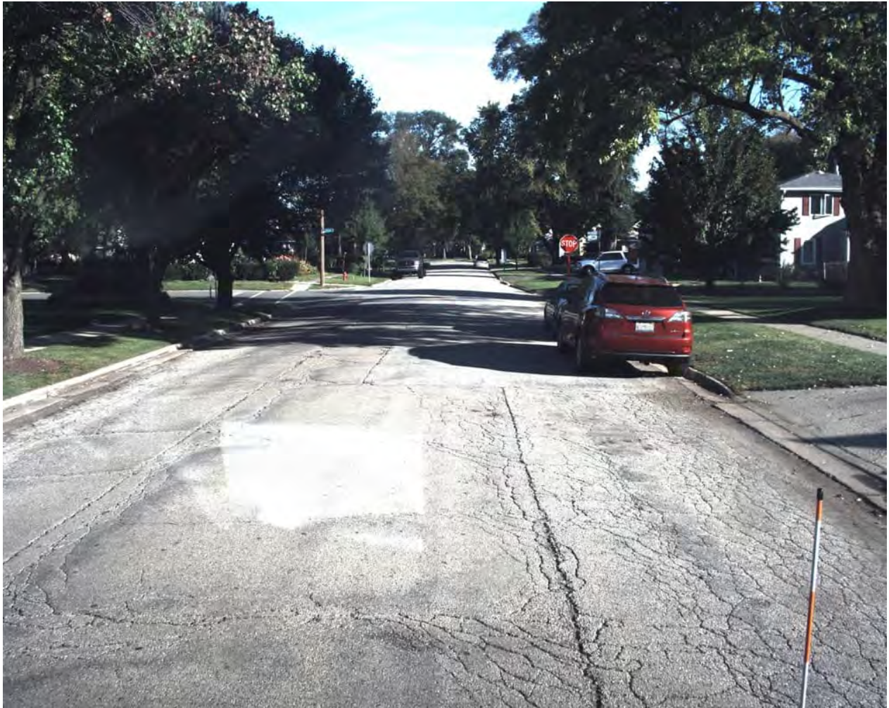
Figure 3-19: Stillweld Dr Section 05 PCI 19 (Serious)
