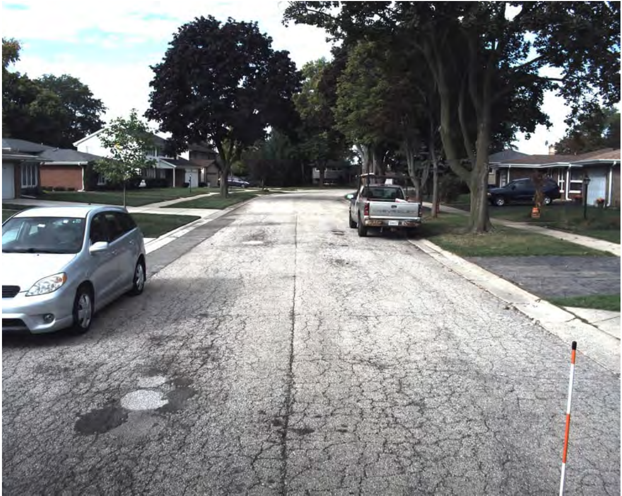
Figure 3-21: Tures Ln Section 00, PCI 10 (Failed)
