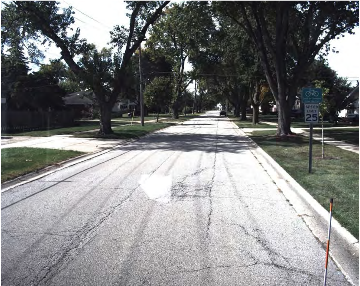
Figure 3-5: Florian Dr Section 00, PCI 50 (Poor)
