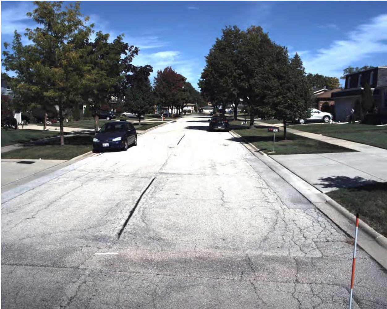
Figure 3-4: Inner Circle Dr Section 00, PCI 55 (Poor)
